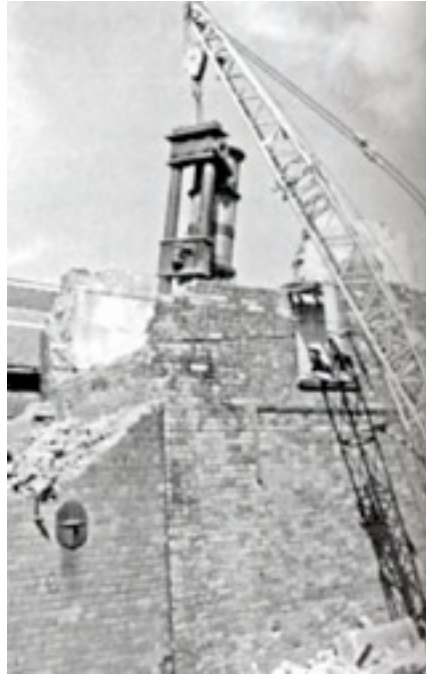
The cylinder of the Haydock engine being removed from the engine house at Haydock.
