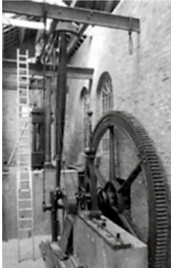
View of the flywheel of the Haydock engine being installed at Liverpool Road.
